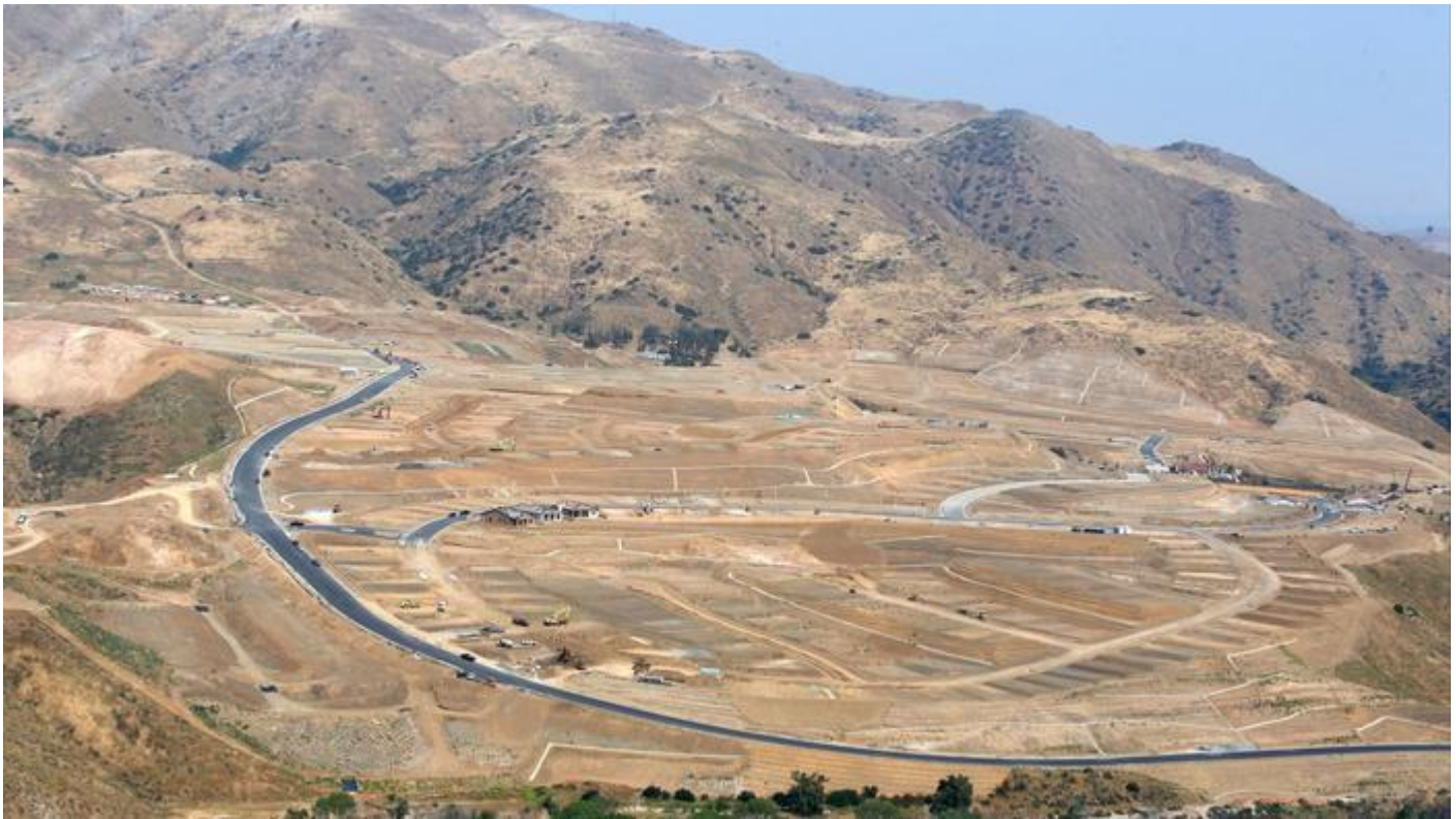
A multi-generational housing development under construction in Temescal Valley. (Christian K. Lee / Los Angeles Times)
